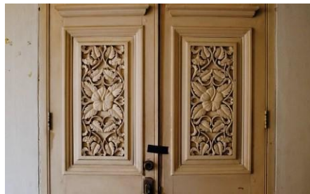
Figure 8. Courtroom doors at Bangunan Sultan Abdul Samad, decorated with local arabesque (featuring the national flower)
